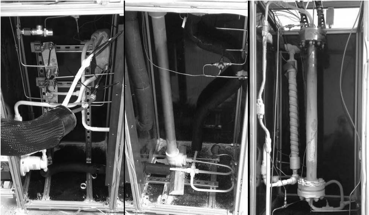
Figure 5-3. Inside view of cold boxes with perlite insulation removed. From left to right: heat exchange and pumping cold box, reservoir cold box, and bubbling heat exchanger and separations cold box
